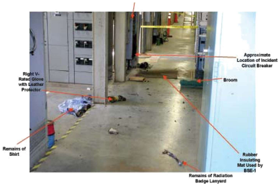
Figure 2-1. Scene immediately after the accident
