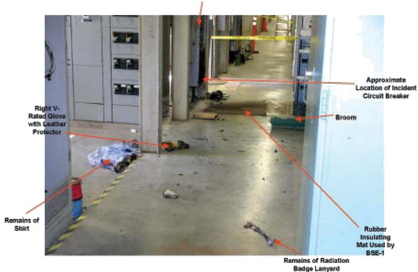
Figure 2-1. Scene immediately after the accident
