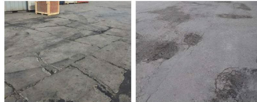
(a) Fatigue cracking in concrete pavement (b) Fatigue cracking leading to surface disintegration
