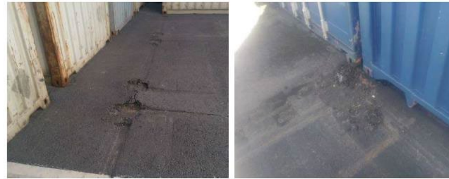
(a) Unstable asphalt (shoving and de-compaction) (b) Unstable asphalt (de-compaction and spalling) Figure 1-7 Un-controlled Deformation
