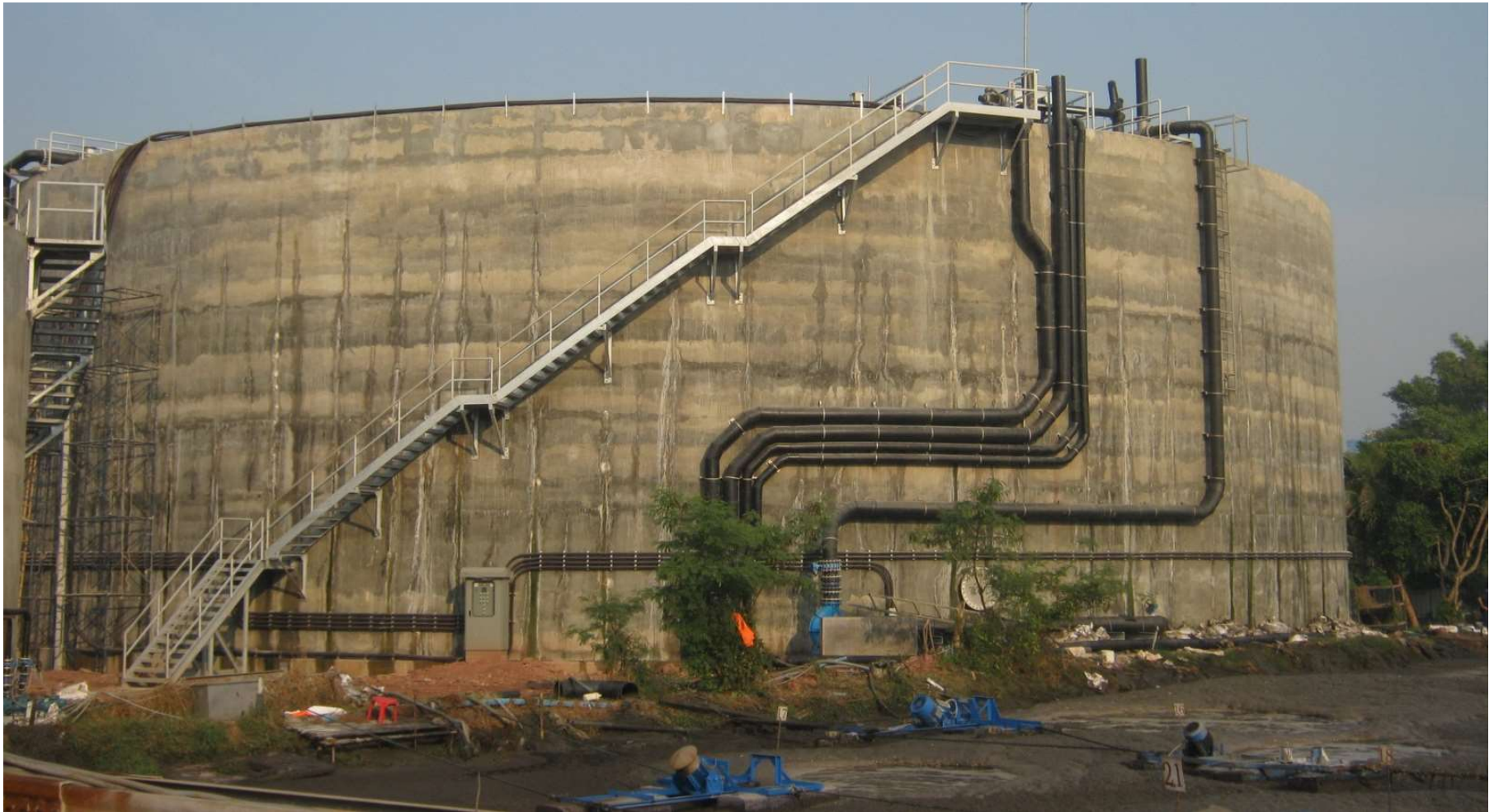
Crack on Waste-water Treatment Plant Wall
