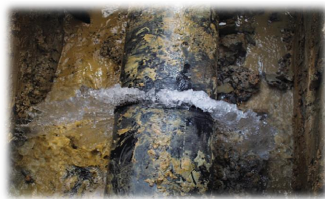
A leak in the legacy water supply infrastructure
