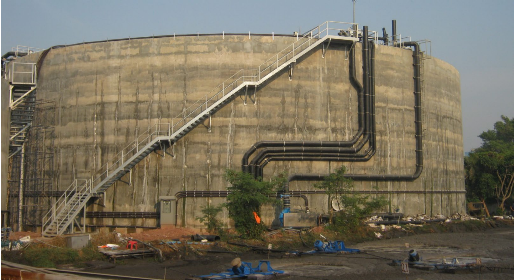
Crack on Waste-water Treatment Plant Wall
