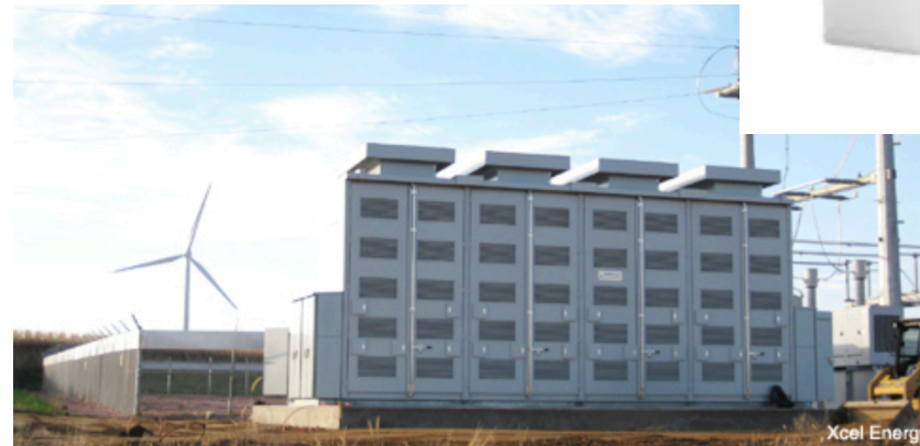
Sodium Sulphur Battery Energy Storage
