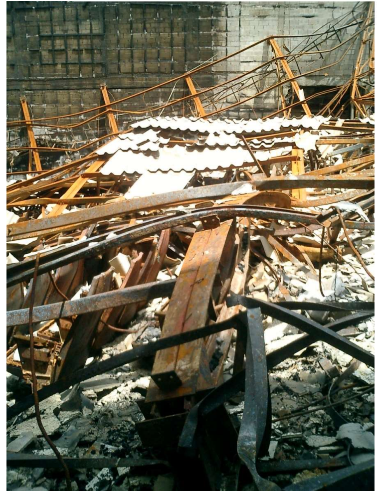
Structural Steel Damage under Fire
