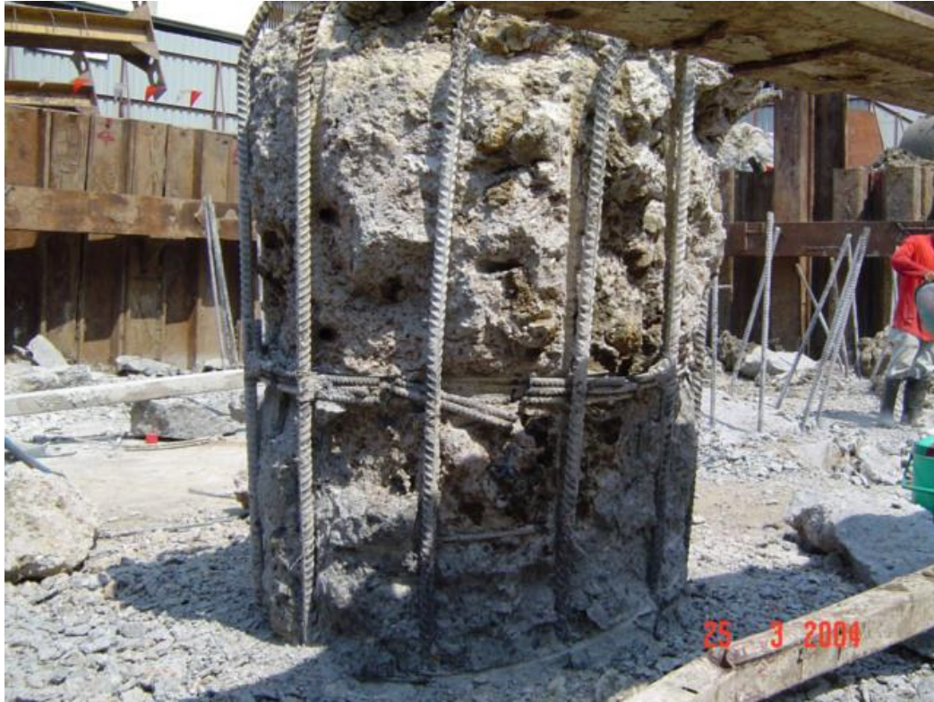
Bad pile head condition
