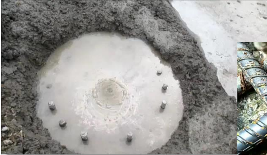
Bleeding of fresh concrete at pile head
