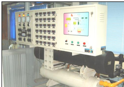
8. Water Chiller Unit
