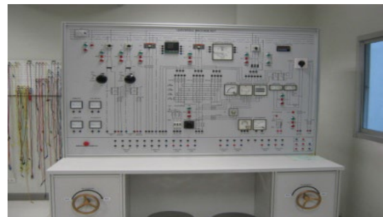
Control Panel for Display
