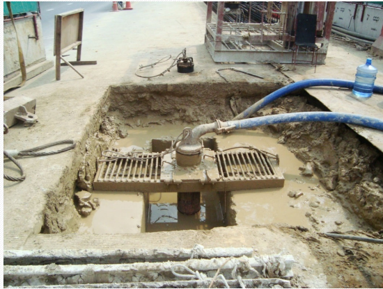
Recycling of drilling fluid
