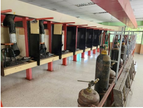
Gas Welding Machines
