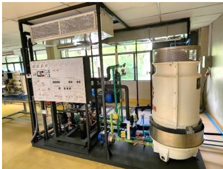
Chiller Air Conditioning Training Module
