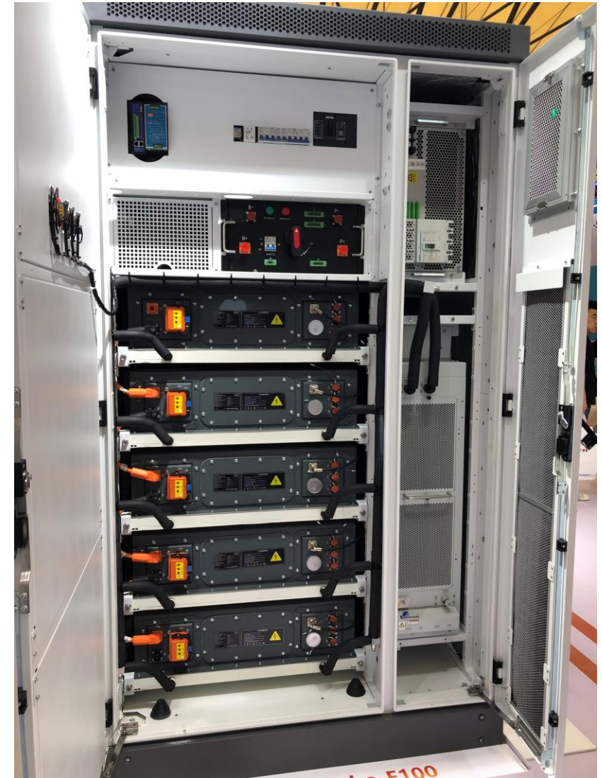
Lithium Ferro Phosphate (LFP) Battery
