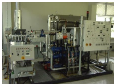
Steam Power Plant
