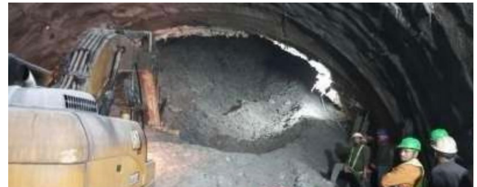
Section collapse trapping 41 workers
