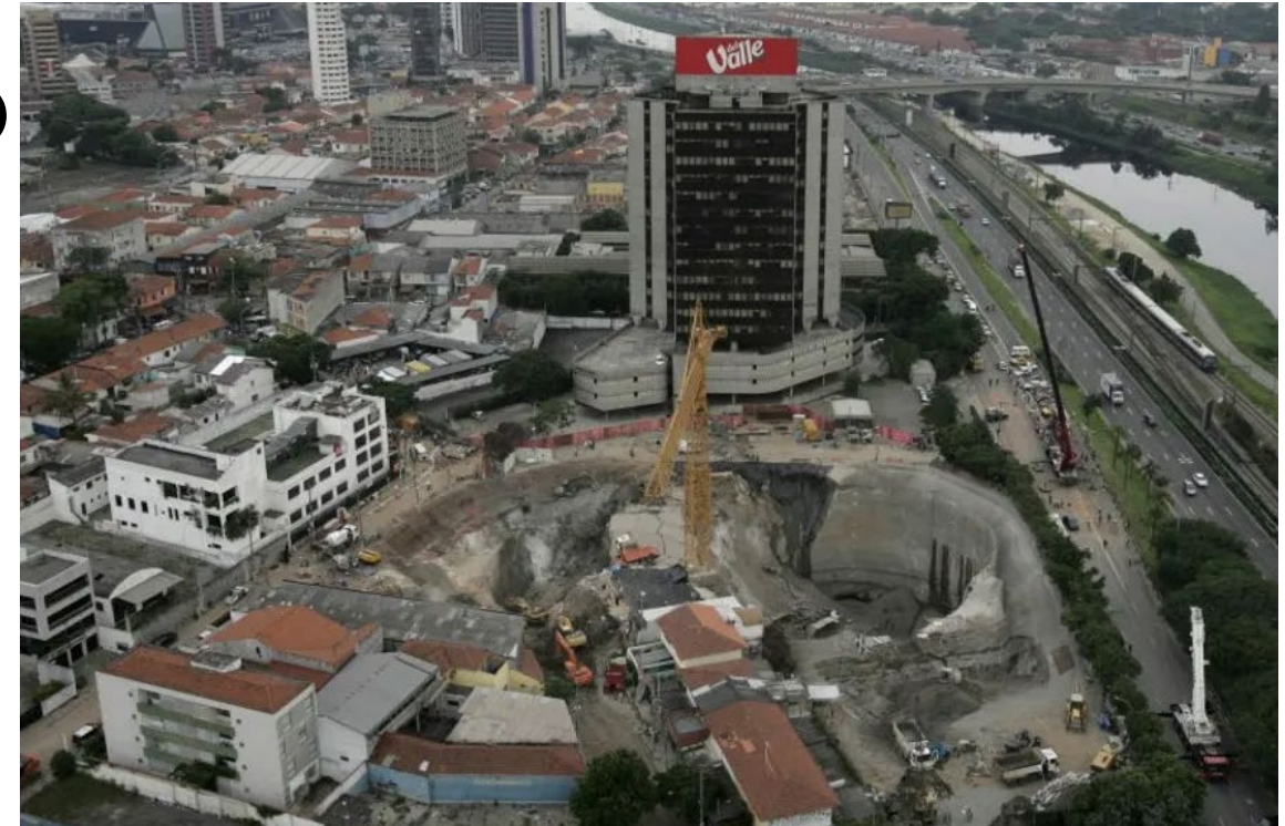
Fig: Drilling in a tunnel to extend the metro system caused a massive sinkhole ,Brazil,2007
