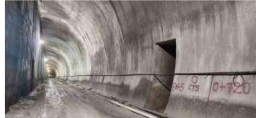
Silkyara Tunnel before the incident
