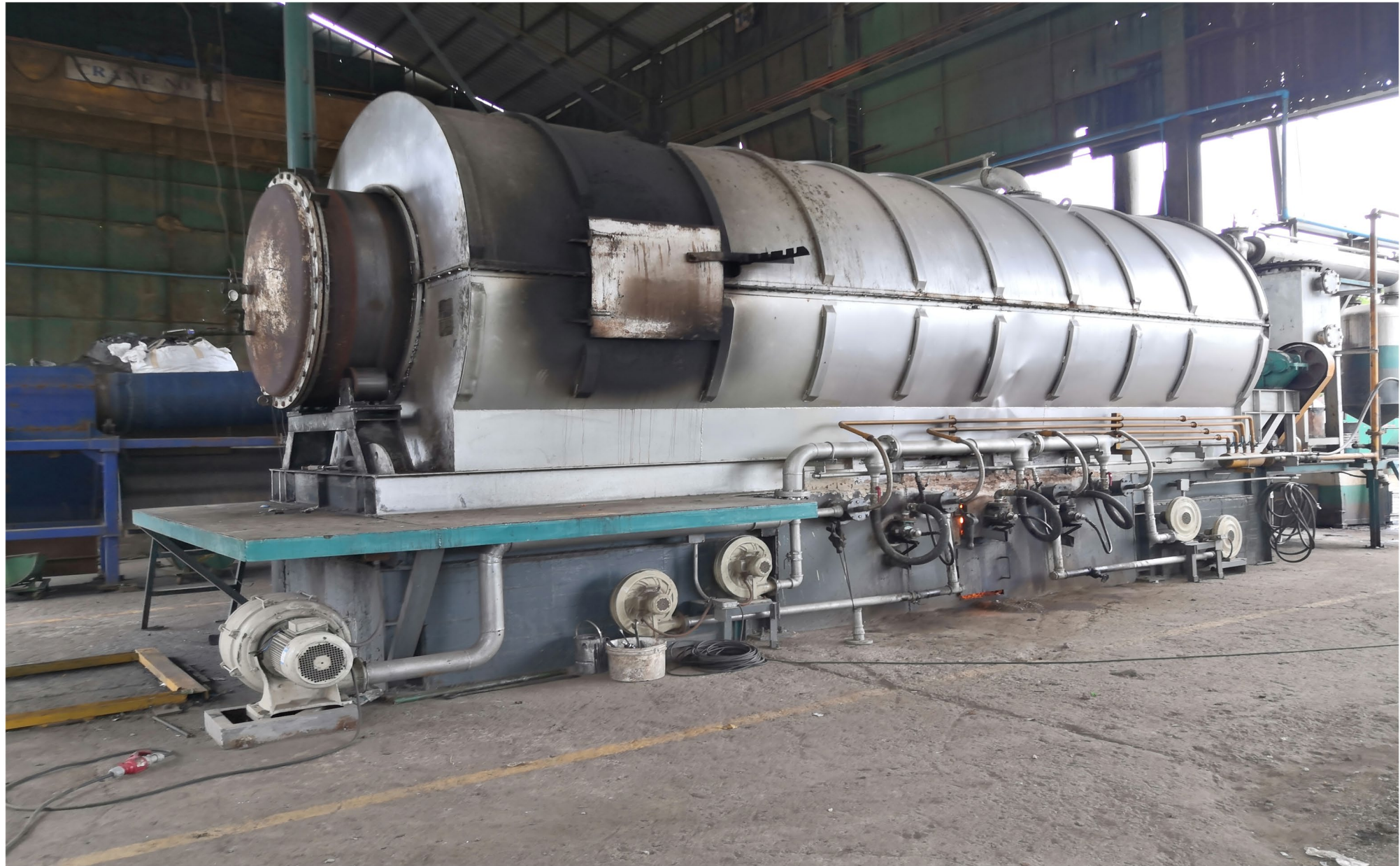
Pyrolysis system – Batch type, 3 ton/day
